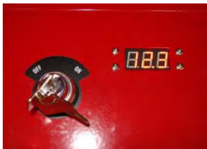
Power Switch & The number show's capacity of batteries
